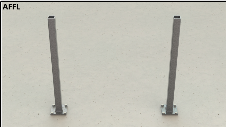
03a) With an Above Finished Floor Level (AFFL) installation you may proceed to the next step.
