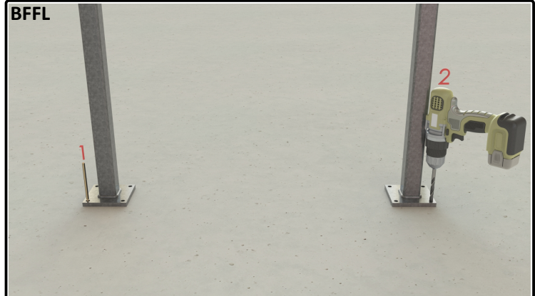
01b) Using your signed off drawings position the primary posts and prepare the structure for fixings.
